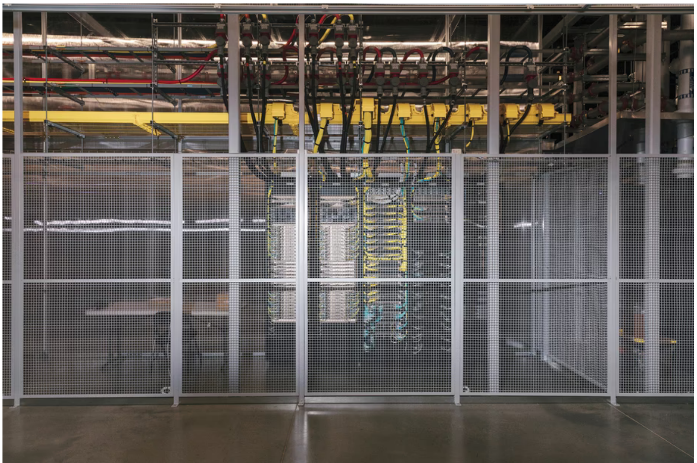
Cabinets of computer chips at a data center in Loudoun County, Virginia (Landon Speers for The Atlantic)
